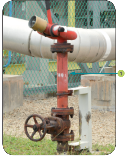
1 Fire hydrant monitor
