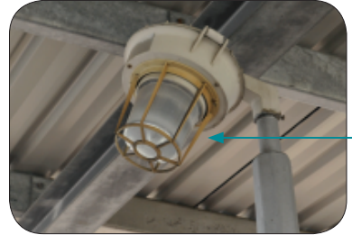
1 Intrinsically safe lighting
