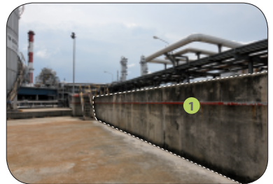
1 Tank farm with bund wall for secondary containment
