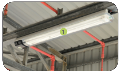
1 Explosion proof light fittings
