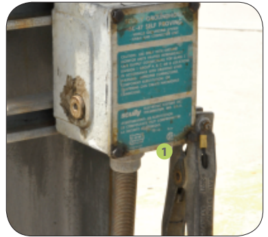
1 Grounding equipment and spring-loaded clip at loading/unloading bay for earthing of static electricity
